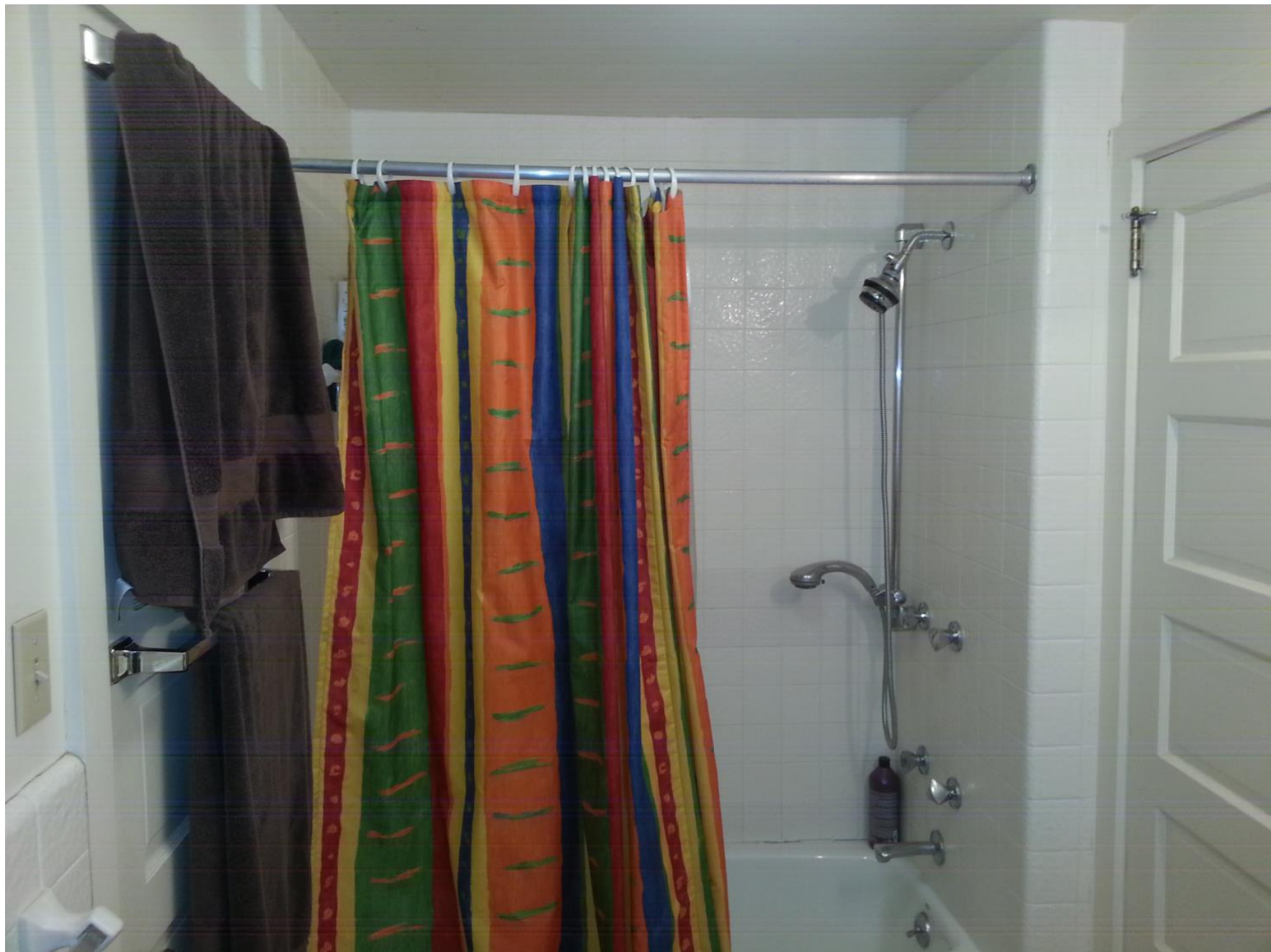
The existing bathroom had a standard 5' bathtub and shower surround. Very plain and uninspiring.
